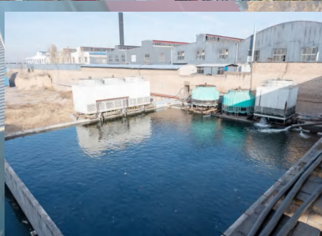
industrial water circulation systems
